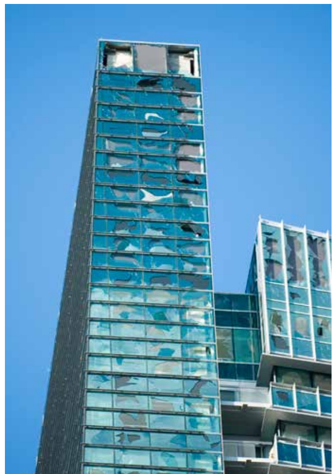
High wind speeds and windborne debris from a hurricane can destroy a building within hours. Damaged bank building at Brickell Avenue due to Hurricane Wilma.
